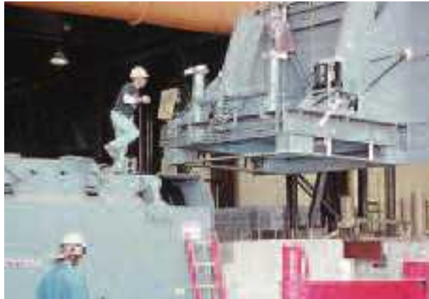
Induction furnace installation in a major foundry
